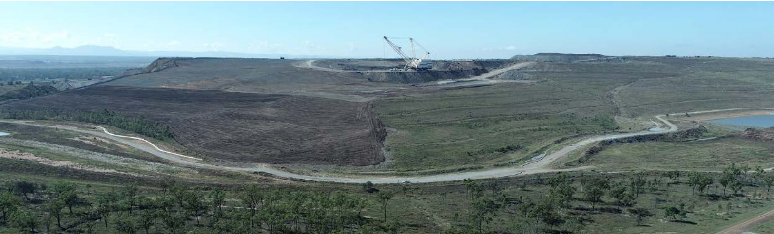
No longer needed for coal production, one of Hail Creek mine's draglines has been re-purposed to shape final landforms.
