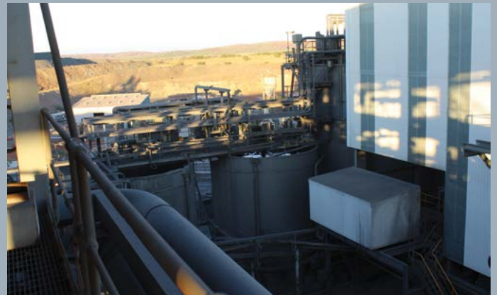
2015 There are now four concentrate storage tanks rather than the original two.
