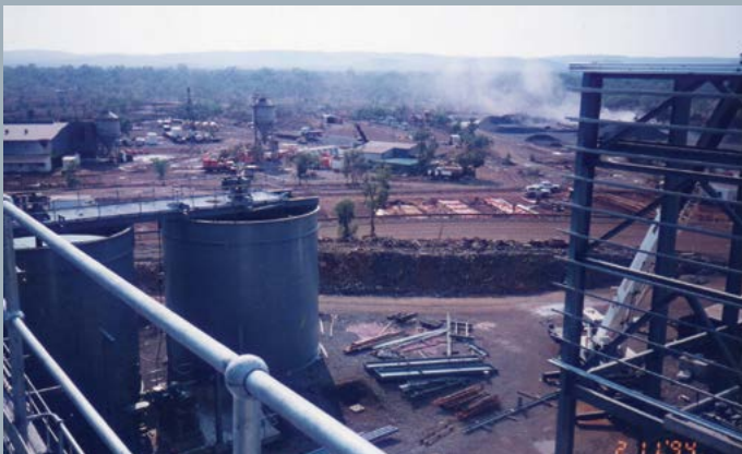
1994 Concentrate storage tanks.
