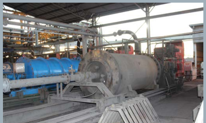
2015 The Isamills are still in operation today.
