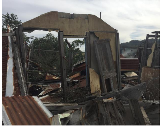
Figure 5 Latter additions to the rear and north of Fairview showing asbestos lining
