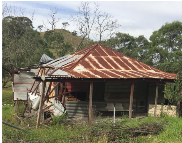
Figure 23 Northern Valley Cottage, the northern verandah has collapsed
