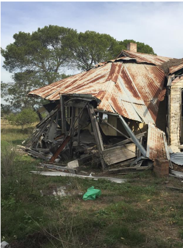
Figure 9 View of collapsing eastern side of Hillcrest
