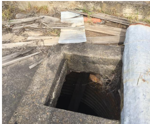
Figure 7 Cistern located to the south of Fairview
