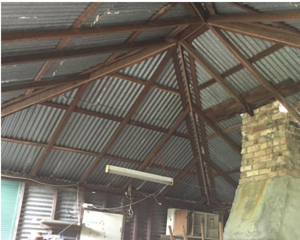
Figure 22 Fire place chimney and interior roof structure at the Northern Valley Cottage
