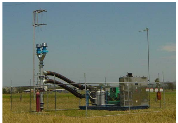
Plate F Operating gas extraction plant
