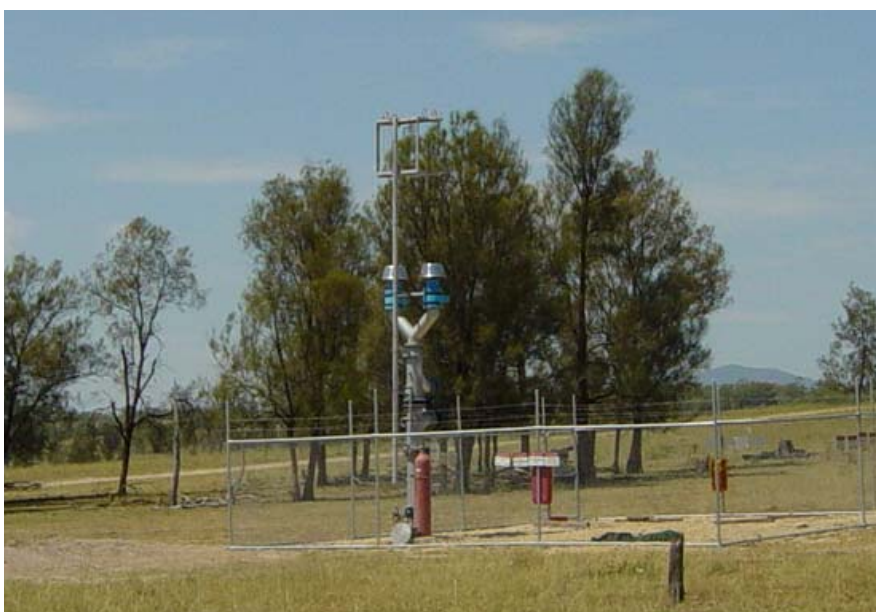
Plate 2.10: A free venting gas drainage borehole assembly. Ref: DSC 00607.jpg
