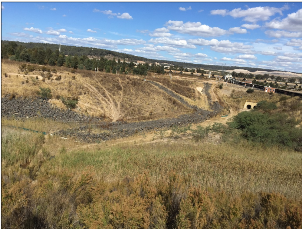
Plate 10 Goulburn River Diversion Pilot Works – Erosion from Kangaroo Tracks
