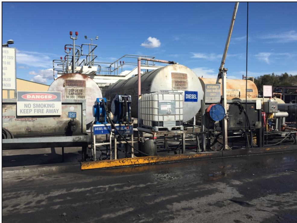
Plate 4 Leaking fuel pump at Ulan No 3
