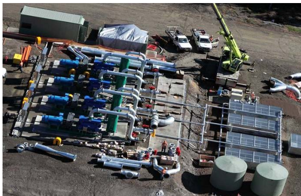
Plate 2.2 – Goaf Gas Drainage Suction Plant
