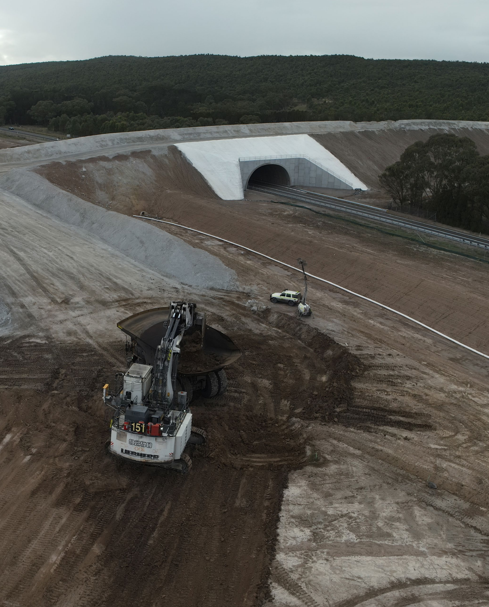
Excavator EXC151 was the first to go over Wybong Road over the new 'Callatoota Pass' on 4th April 2024. The name of the overpass was determined through a naming competition at the mine – everyone agreed this was a clear winner as a nod to the history of the area – the site of the former Callatoota Estate vineyard. In the background, the vegetated hill is an example of our mine rehabilitation.
