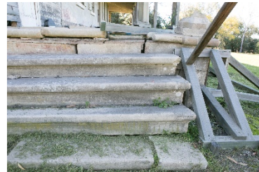
Image 06 New House: south west corner, further collapse now evident.
