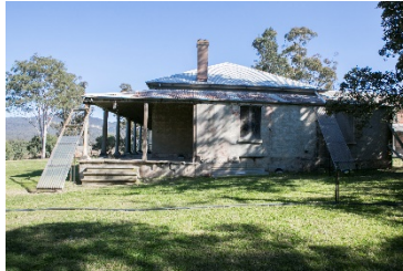
Image 02 New House: east elevation. Water ingress.
