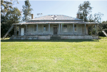
Image 01 New House: south elevation. Verandah stone work failing and roof dropping.
