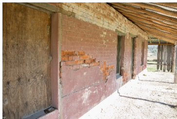
Image 23 Stud Masters': Extensive clean up and stabilisation. Brickwork failure.
