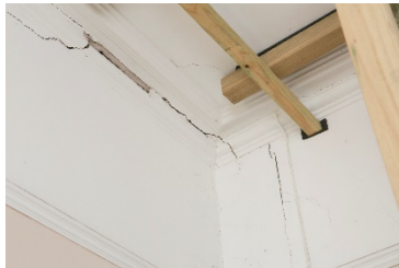
Image 05 New House: propping for temporary stabilisation has been installed. Obvious cracking.
