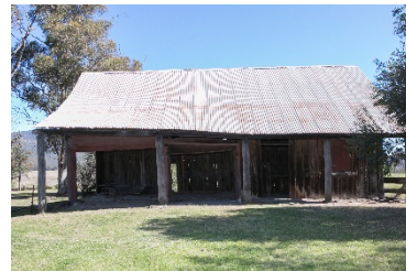
Image 21 Carriage House: requires temporary building bracing.
