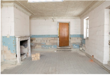
Image 13 Kitchen Wing: Interior. Dust in piles from decaying walls.
