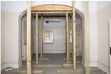
Image 04 New House: recent interior propping. Extensive cracking evident.
