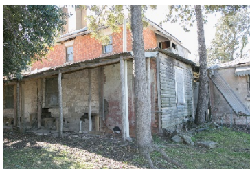
Image 11 Kitchen Wing: south west corner. Water ingress, supports missing, close trees.
