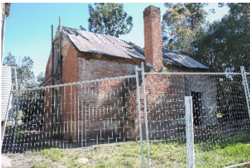
Image 19 Servants' Wing: salt attack obvious, roofs gone, roof failed, stairs missing. Brickwork failed.
