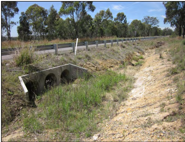
Figure 38: Three pipe concrete culvert and modified ditch at the southern end of the proposed realignment at MGA 318886/6381856 (IMG 1493).
