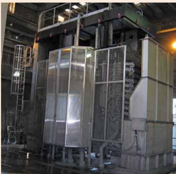
The new Larox Filter 1 is now installed and operational at the Mill.
