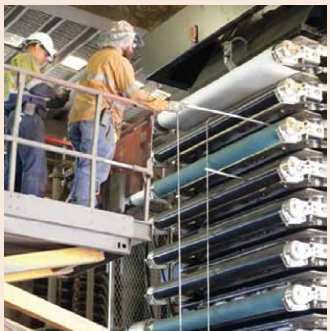
Filter cloth is installed on the new Filter 1 by Jim Rego from Outotec and Scott Walter from Blue Sea Cranes.
